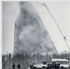
The demolition of the seventeen-story high Skrunda Radar on May 4, 1995. Image: Alisa Jermaks
